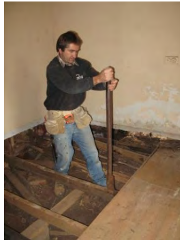
Right - Will Cass lifting the floor boards in the soon to be archival room (back room)
